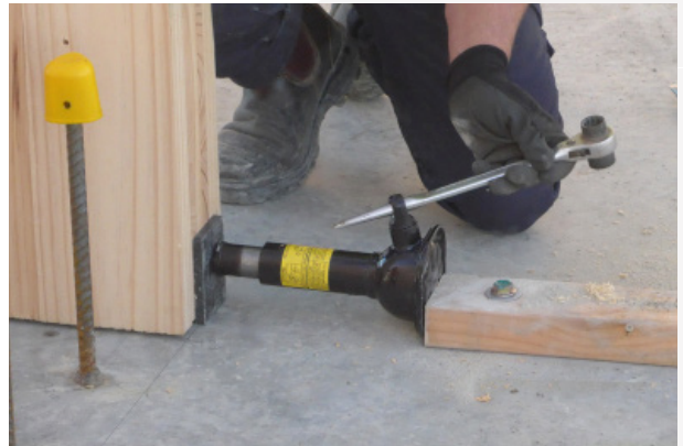
Jacking from a bolted floor anchor to tighten a joint or take out edge bow.
