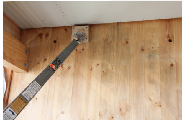
Non-breathable building wraps promote surface fungal staining.
