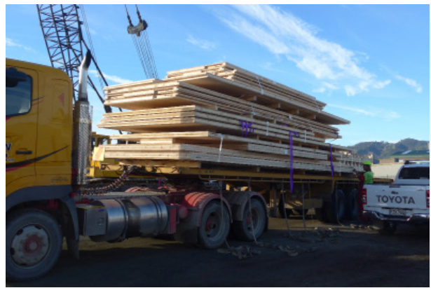
Packs are strapped to pallets ready for lifting off at the site.
