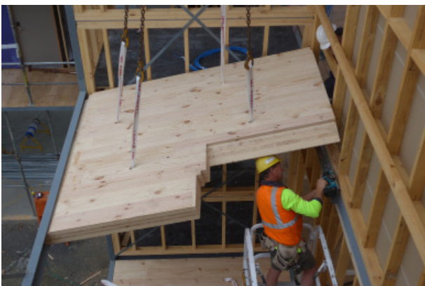
The upper PFC flange impedes placement of a stair landing.
