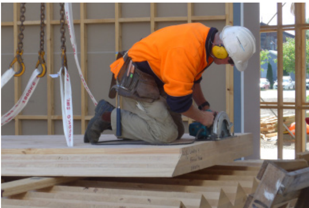
Insufficient tolerance leads to time lost in site trimming.
