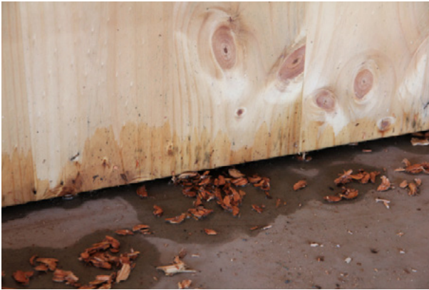
Ponding water migrating into unprotected end grain.
