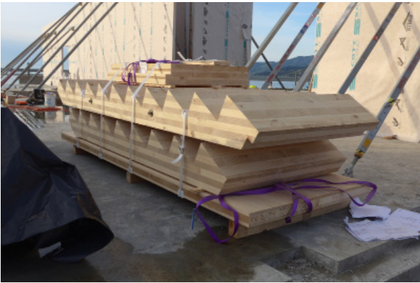
Even pack support well clear of the floor slab.
