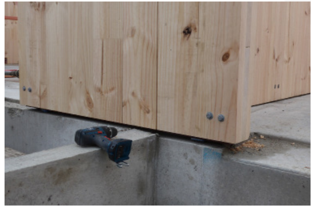
Clearance from the concrete floor slab prevents moisture penetration.
