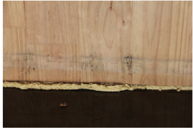
Water stains can be difficult to remove.
