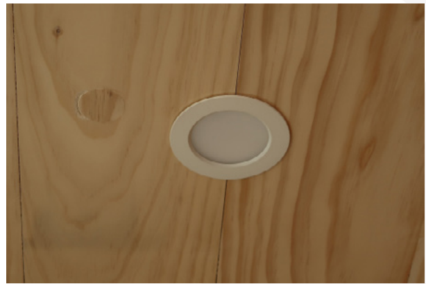
Edge crushing has required some repair around the plug.
