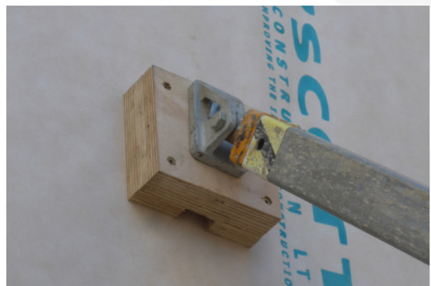
The wrap and a timber packer properly protect the Natural Appearance Grade surface.
