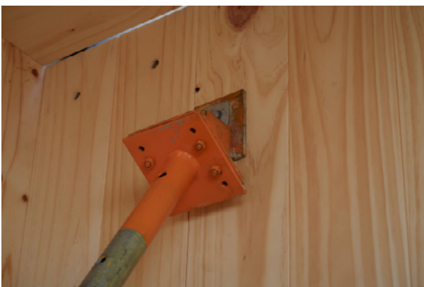
Construction moisture reaching this connection will stain the surface.
