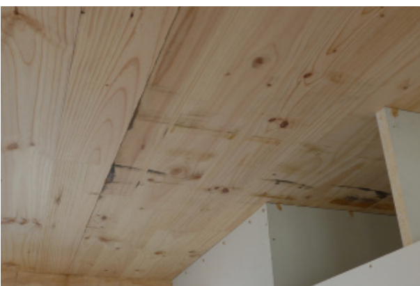
Natural Appearance Grade surfaces damaged by poor storage and handling.
