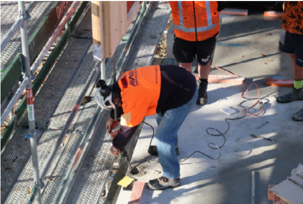
A setout error requires remedial work with the panel held in suspension.
