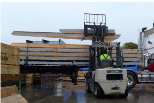
Panels are vulnerable to forklift damage.
