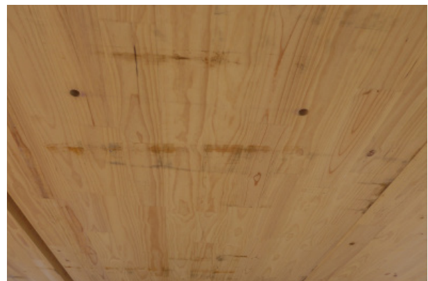
Marking by unprotected forklift tines.
