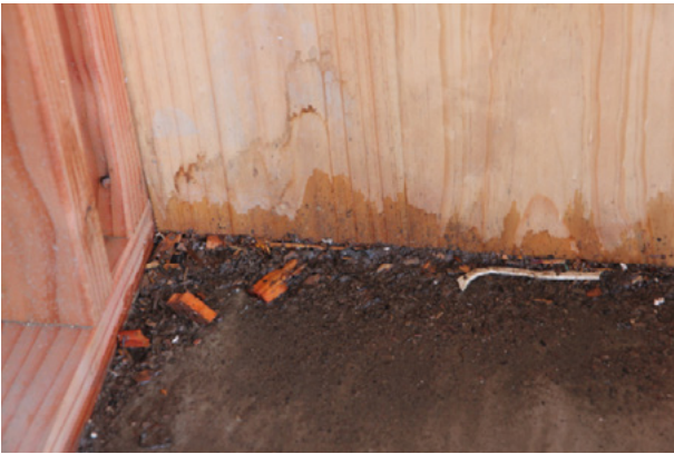
Keep walls clear of moisture-accumulating rubbish.
