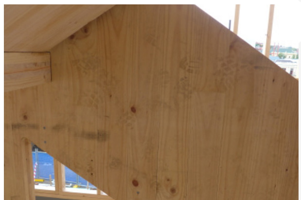
Disfigurement from contractors walking on uncovered panels.
